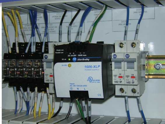
Allen-Bradley standard devices throughout the control enclosure to facilitate local sourcing.
