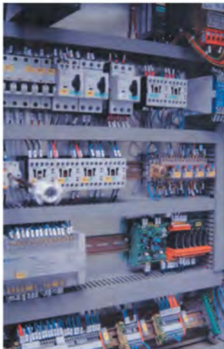
Electrical Box with Numbered Wires This set-up also allows for wiring in options at a later date
